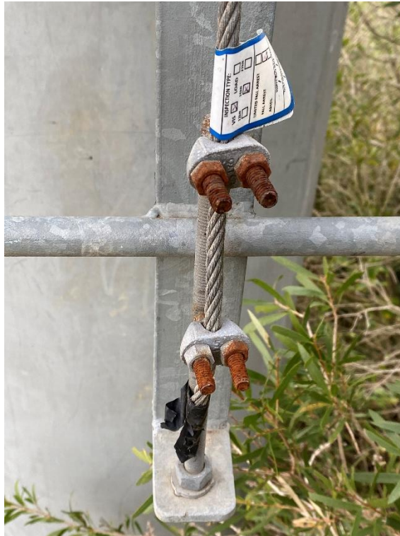
Photo 16 – Corroding wire grip 'U' bolts.
