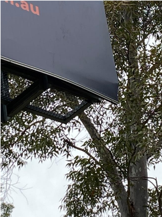
Photo 18 – Deformation to signage pan.
