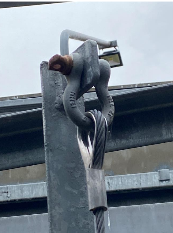
Photo 15 – Corroding shackle bolt.
