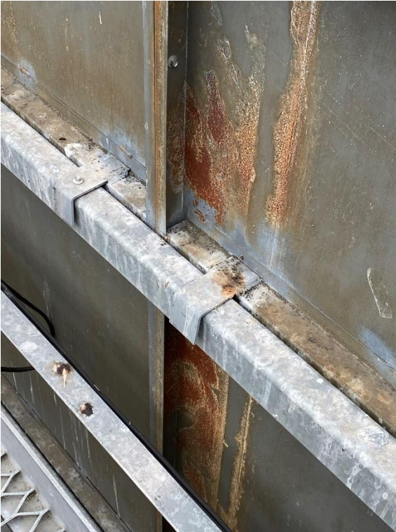
Photo 14 – Minor surface corrosion to signage pan.
