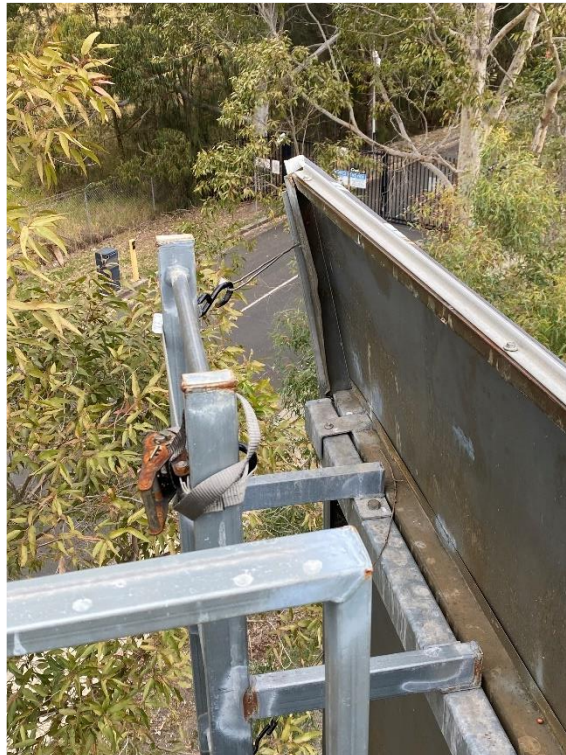
Photo 17 – Deformation to signage pan.
