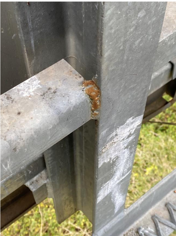
Photo 11 – Minor surface corrosion to welded connection.
