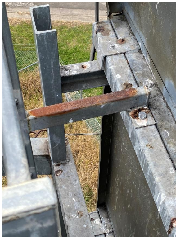
Photo 13 – Surface corrosion to vertical ladder support framing.
