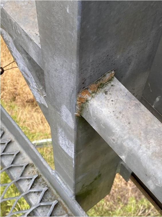
Photo 10 – Minor surface corrosion to welded connection.
